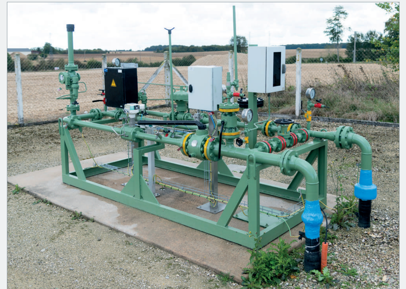
NaTran pressure reduction station.
